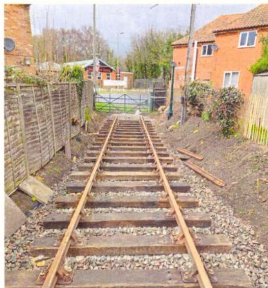
ABOVE The present end of the line, at the junction of Buller Road and Station Road. Leiston station is just behind the trees in the background. LWR
