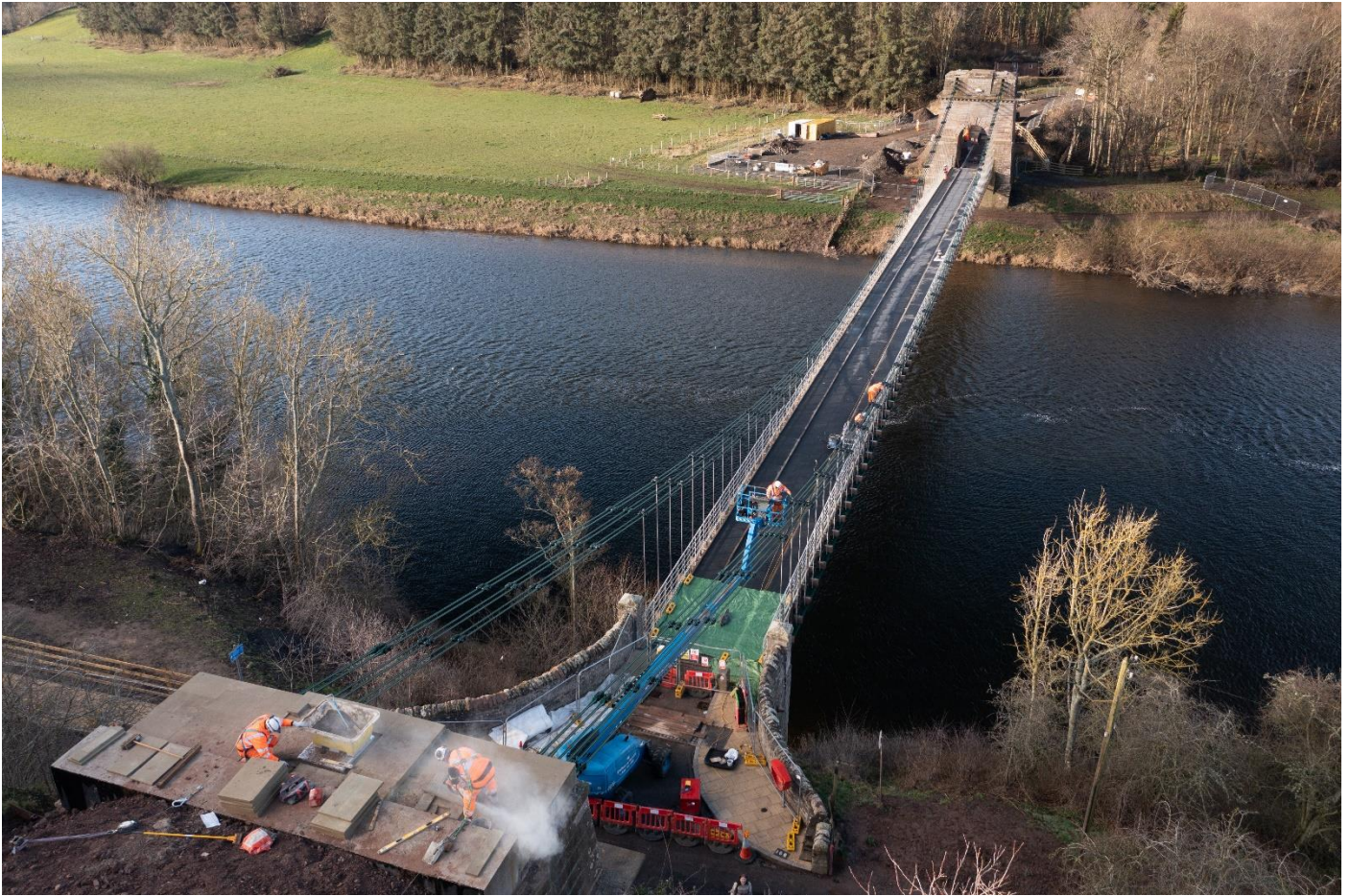
2 nd March – Engineers work on the top of the English tower, bottom left, while painters carry out snagging work from a cherrypicker and the footway.
