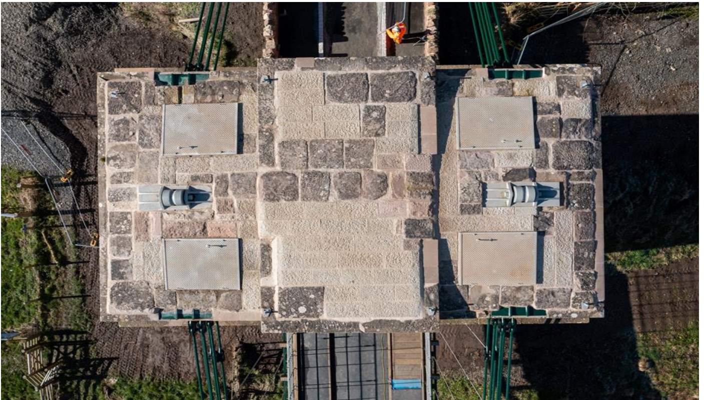
A drone's eye view of the top of the Scottish tower, showing the restored roller mechanisms, now redundant after the removal of the 1902/3 wire ropes, left and right; the four chain inspection covers are also prominent.
