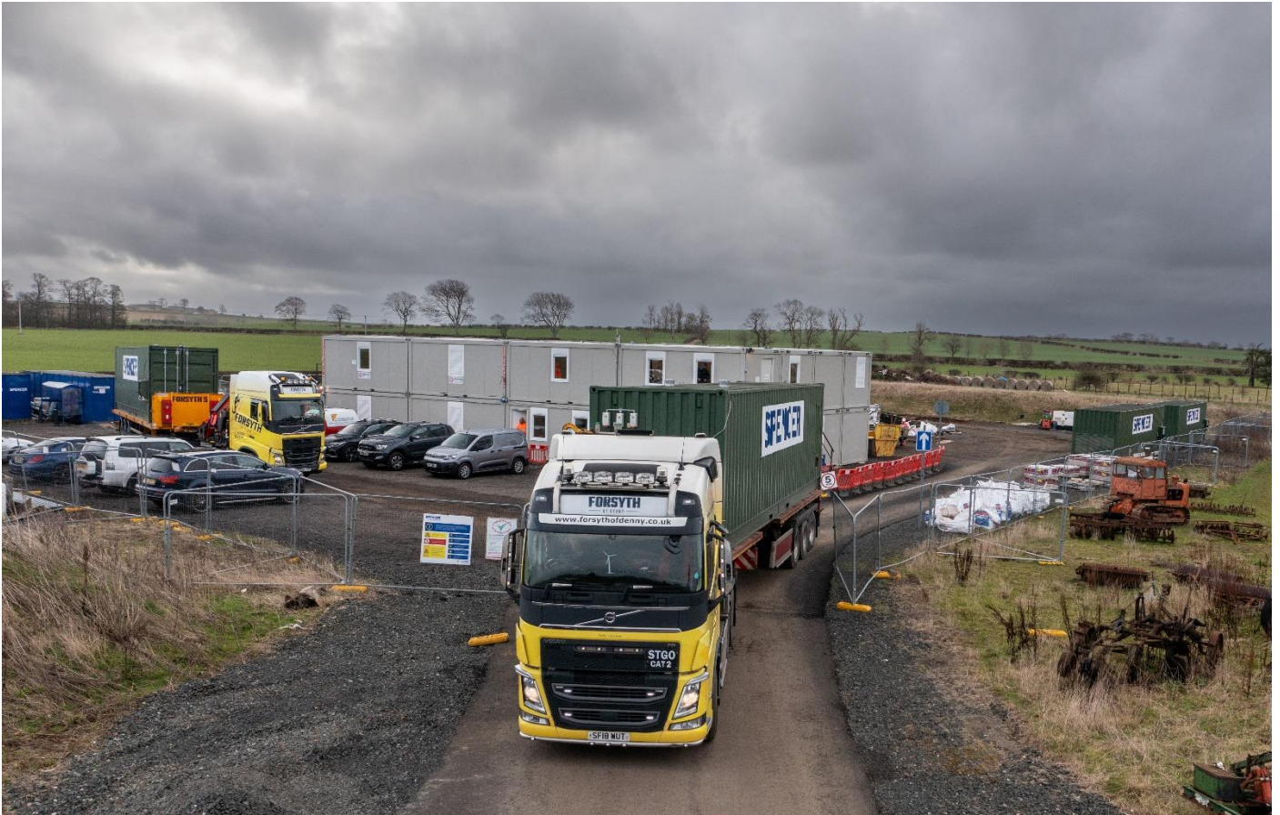
27 th February – under an ominous sky, dismantling of the Spencer depot begins, with the removal from site of the paint shops.
