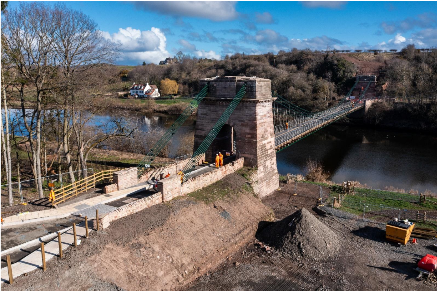
Scottish-side Bridge approach, with new road and footway configuration, restored stone walls, site compound bottom right, and the entrance to the north-side riverside footpath – yellow fence – middle left. The parking layby is just visible adjacent to the half-constructed fence bottom left.
