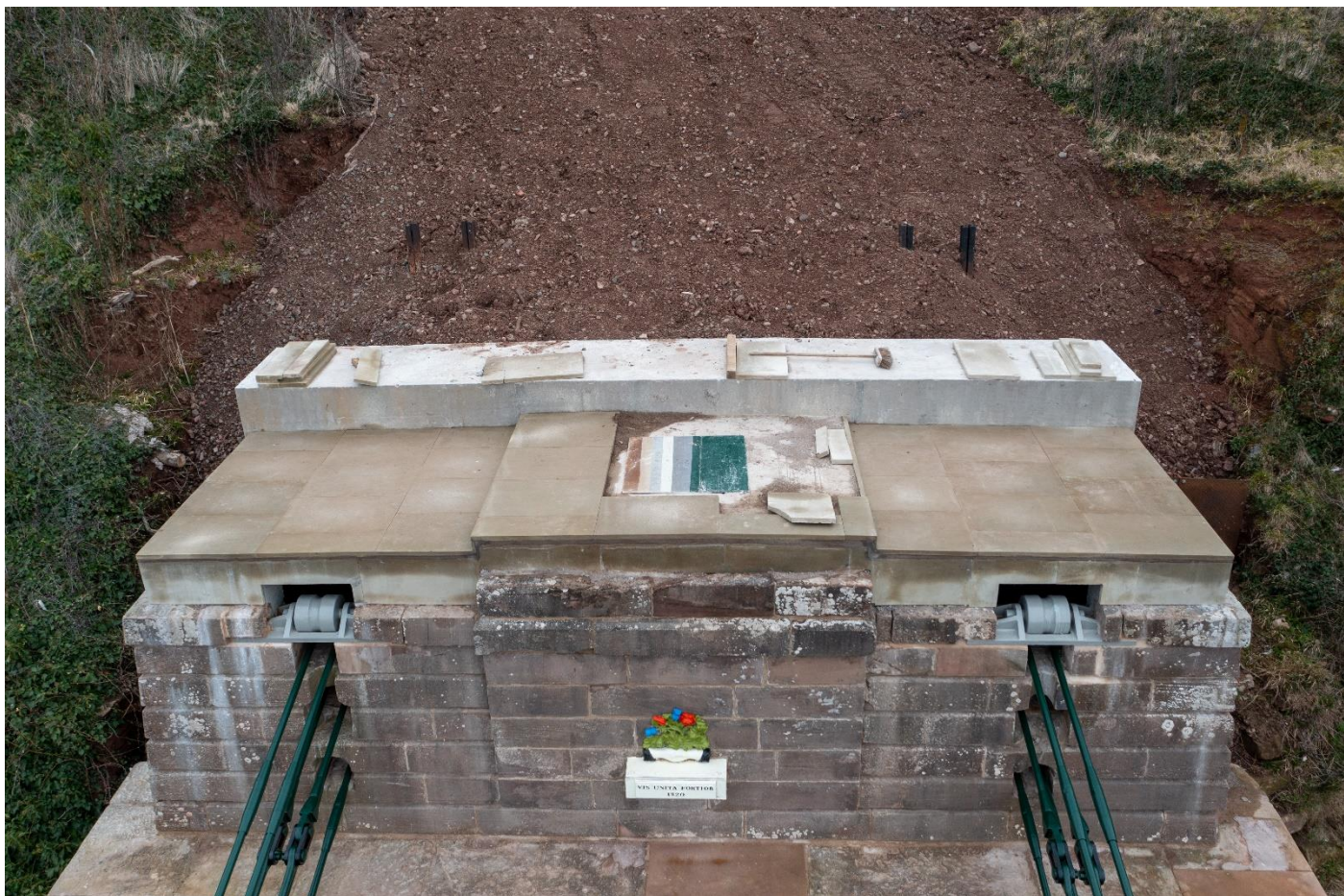
27 th February – Paving of the surface of English tower in course of completion, with the restored Vis Unita Fortior plaque below; also below.
