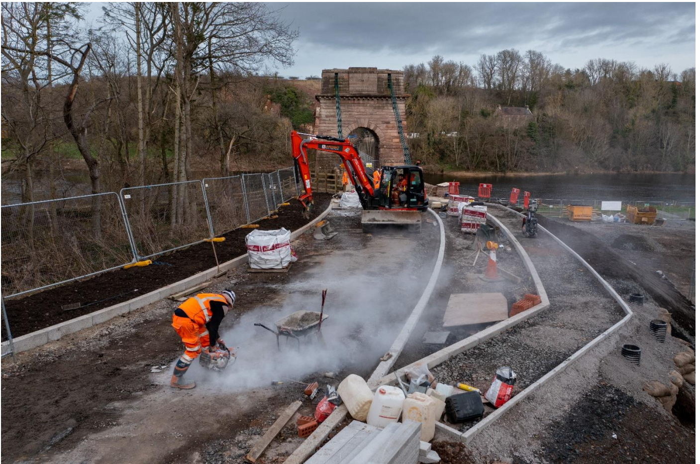
23 rd February – the new Scottish-side road and footpath configuration takes shape, with the parking layby prominent, centre-right.
