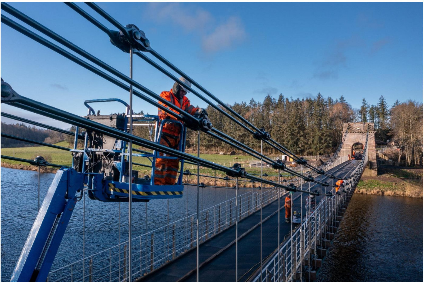
2 nd March A painter working from a cherrypicker inspects a chain link assembly prior to remedial painting, while colleagues work on lower-level snagging from the Bridge decking.
