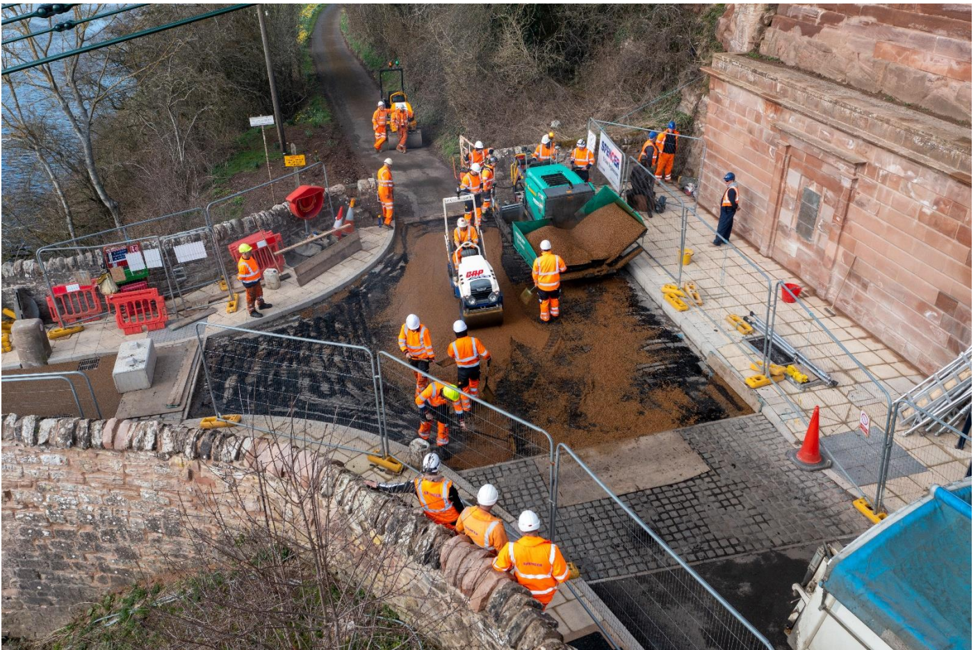
21 st March – A hive of activity on the English approach as contractors lay distinctive buff tarmacadam. Samuel Brown peers out from behind the Spencer sign.
