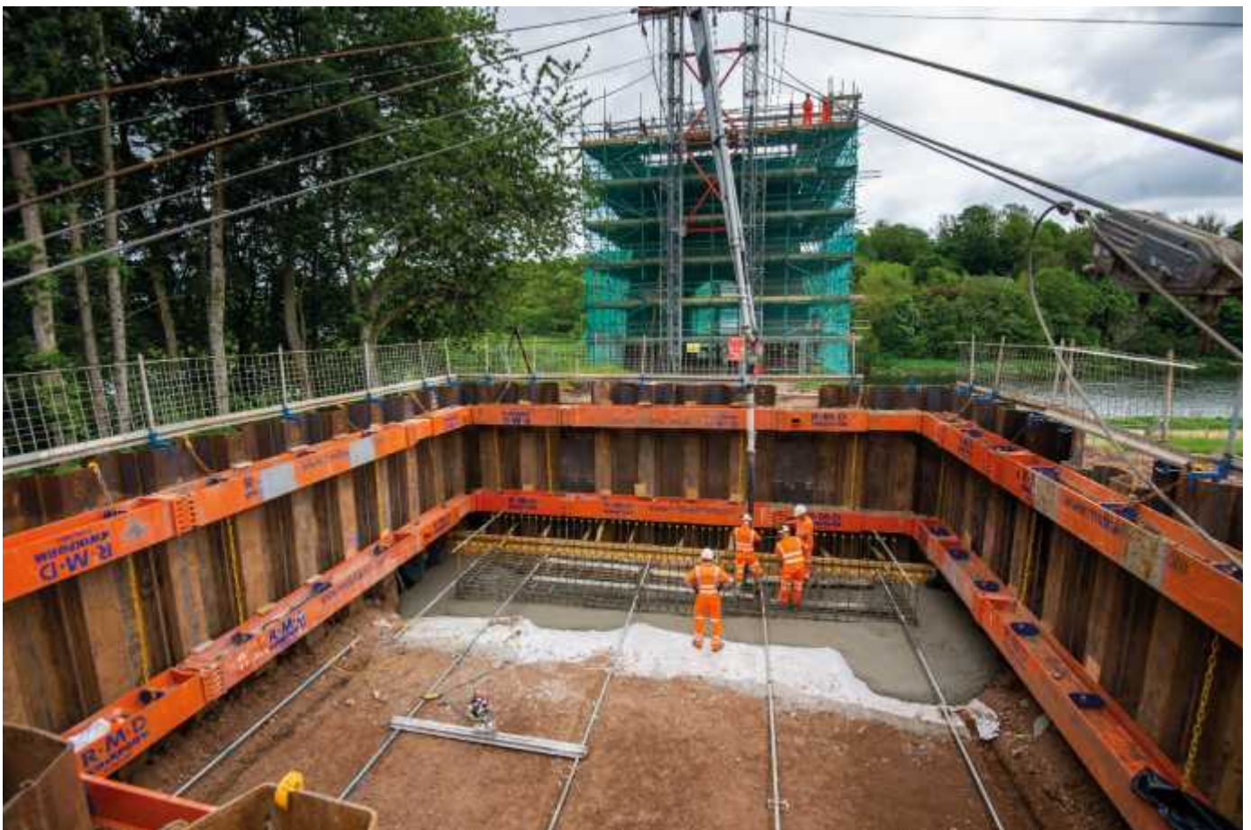
The first concrete pour into the massive Scottish-side anchor block. See following page.
